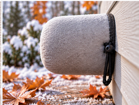
Hose disconnected · Bibb covered
